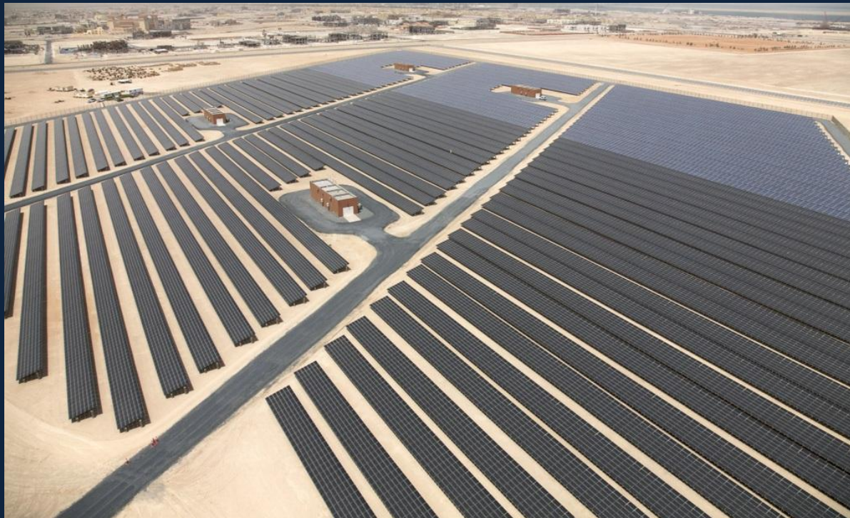
Example 10 MW p PV power plant installed by CH2MHILL for MASDAR in Abu Dhabi (2009)
