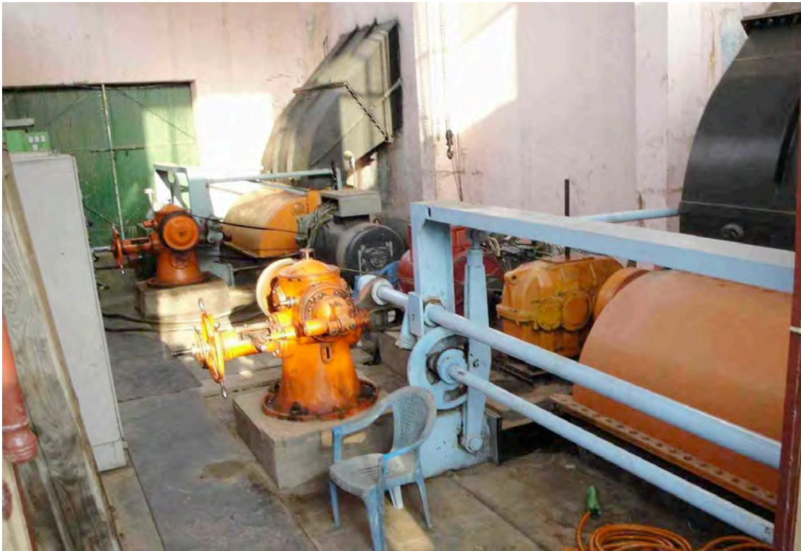
Fig. 4. Asad-Abad powerhouse with 2 crossflow turbines producing ~185 kW each.
