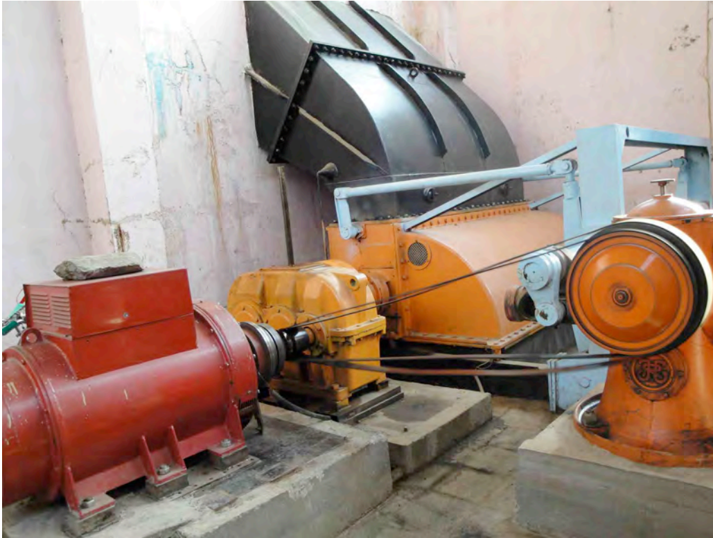
Fig. 5. Asad-Abad turbine and generator (notice rock on top). The system should be rehabilitated to double production back to the original 700 kW power rating.
