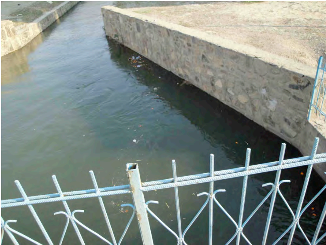
Fig. 7. Asad-Abad canal intake for the MHP station.
