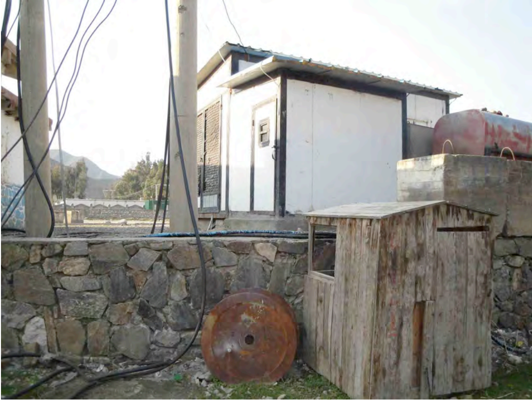
Fig. 6. Asad-Abab MHP power house and transmission distribution.
